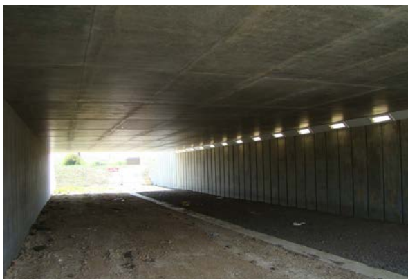
Tunnel showing lighting
